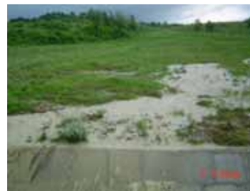
Cerna drenuri blocate
